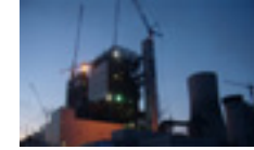
Bulgaristan Mantza East-1 Termik Santral
